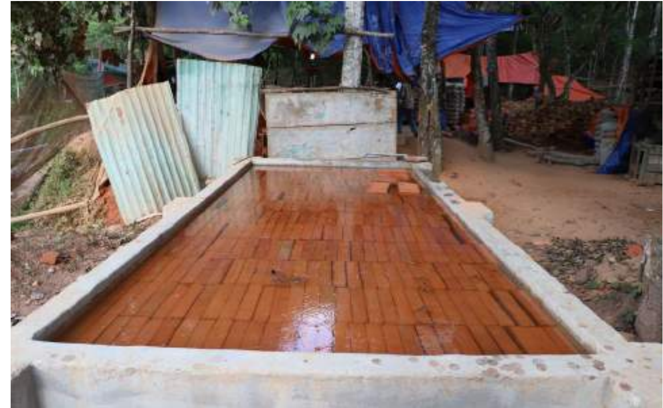
Brick Soaking tank
